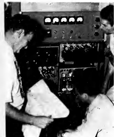
Engineers at WTVR, Richmond tele outlet, check the installation of new transmitter equipment. Station plans to be on by late 1947 or early '48.
